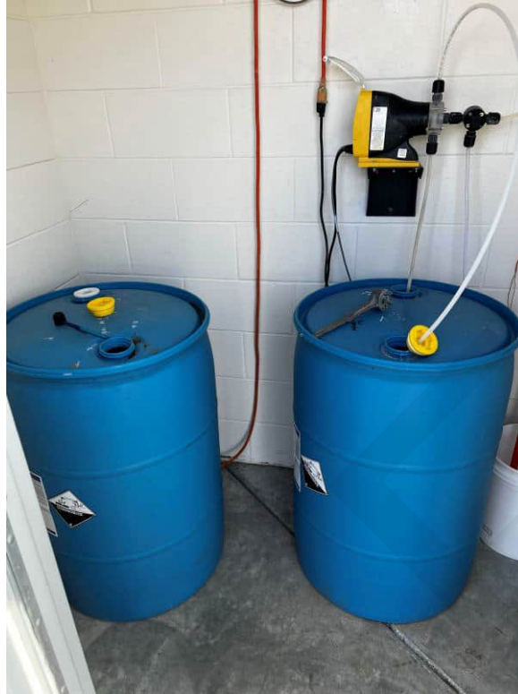
Figure 2-29 Liquid Chlorine Storage Tanks
