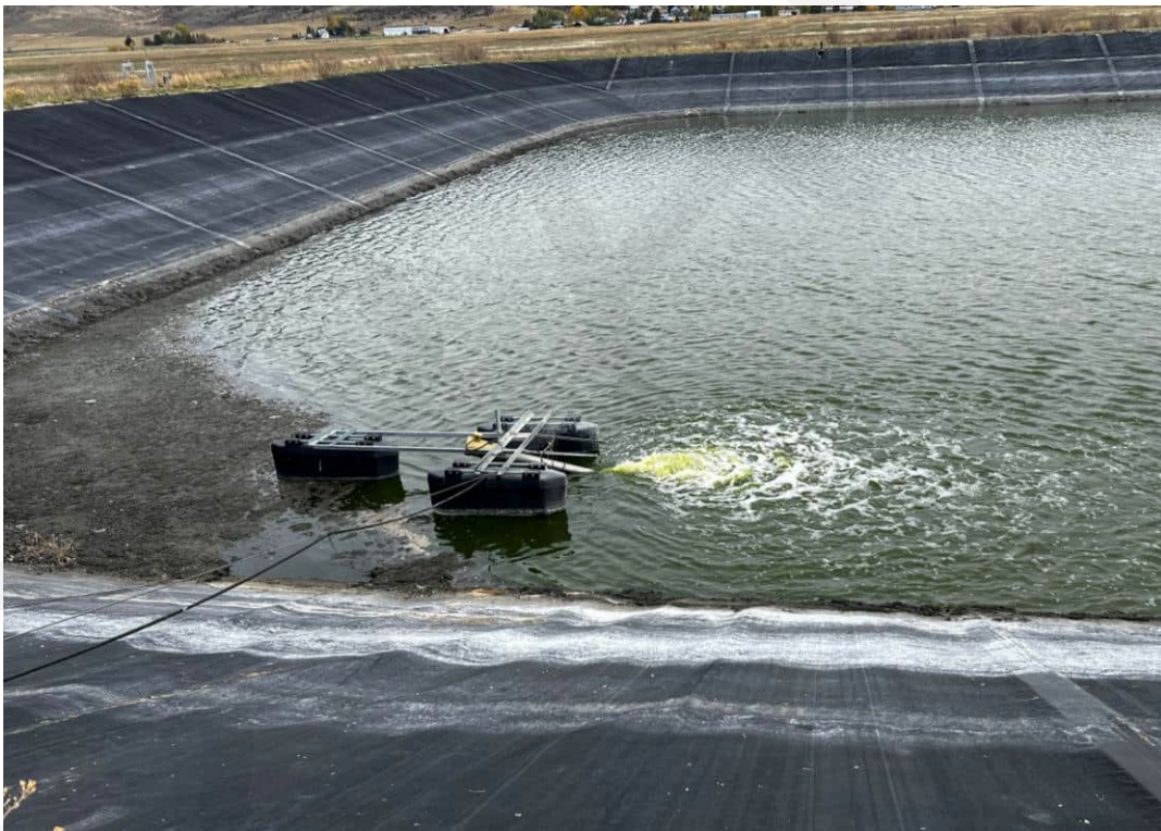
Figure 2-22 Aerators in Lagoon Cell 1
