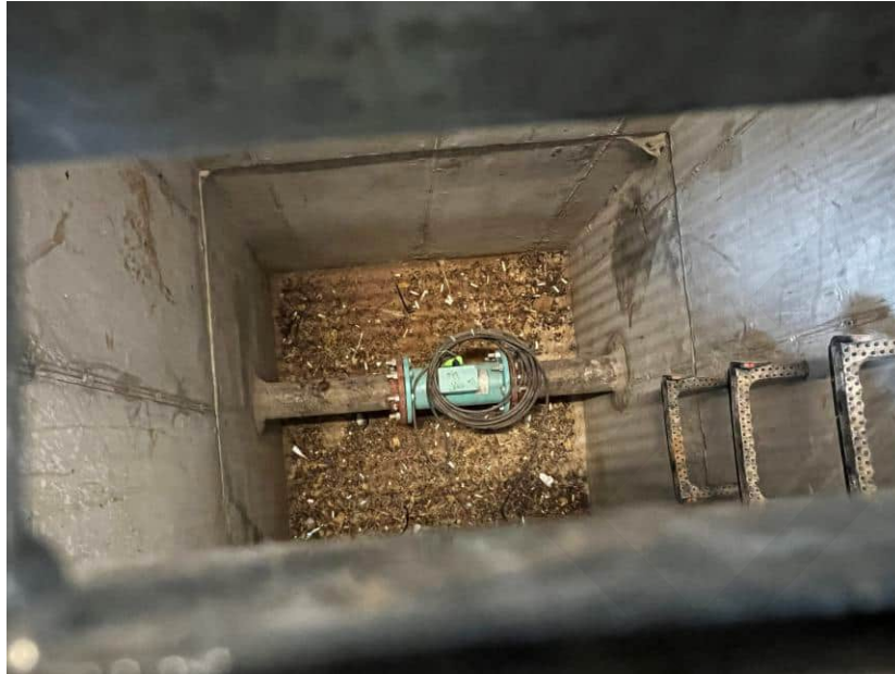
Figure 2-18 Flow Meter in Control Building
