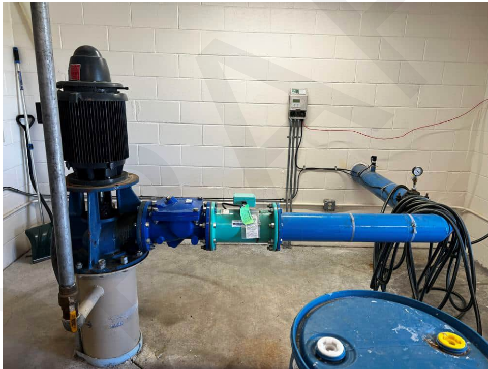
Figure 2-28 Vertical Turbine Pump and Flow Meter
